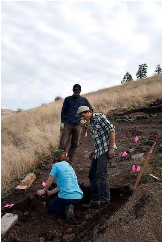
Mario Colucci and Matt Dunkle look at Billy Janczewski (son of RWM's member) helping out with the digging. Mario and Matt were the main engineers of the step structure built this day. Step structures have been built at about half of the switchbacks on the Missoula's most popular trail.
